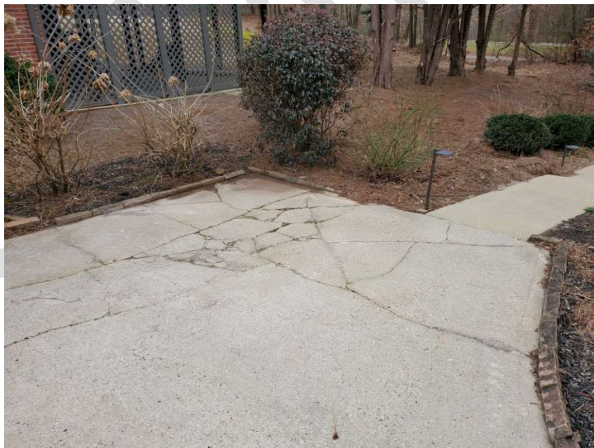
< Fig. 3 – Cracks at driveway >
