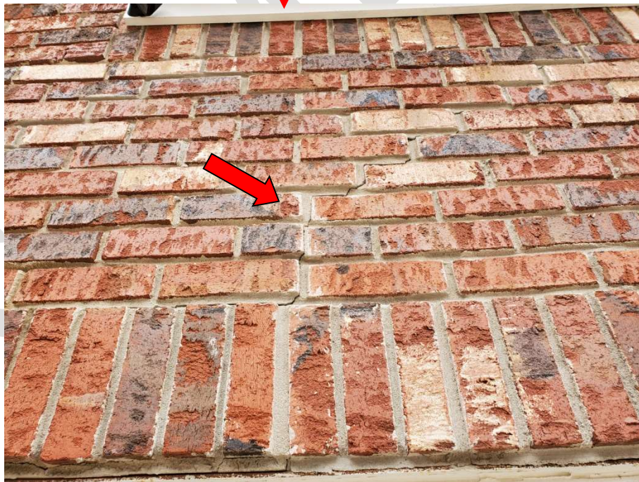
< Fig. 2 – Step cracks at brick veneer >
